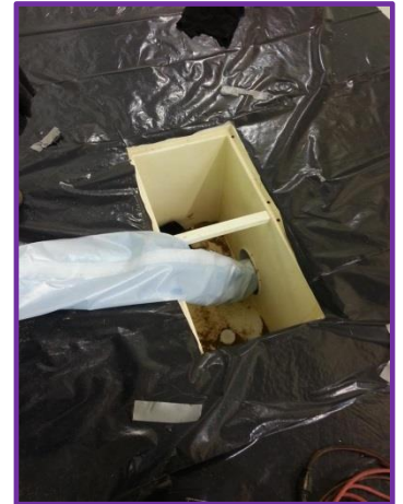
8” main drain in Activity Pool
